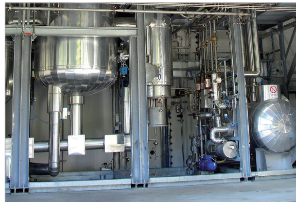
Interior view of the SYNTROL® plant
